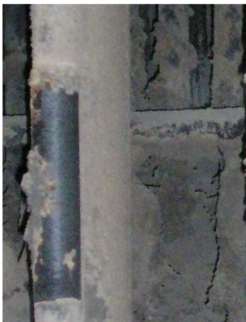
Fig 5: Boiler tube shield with baked-on high emissivity coating after 3 months of service. There was no change in appearance after 9 months service.
