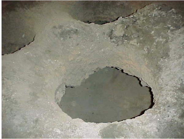
Fig. 6: Precast delta with high emissivity coating after approximately 2/3 of its service life. The delta was put back into service, where it provided over 100 additional heats.
